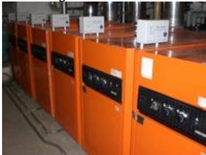
M2G Installation IMechE
