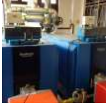
#10 M2G Installed across #5 buildings
